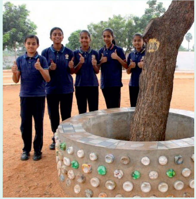
Demonstrating practical application of the 3Rs by constructing a retaining wall around a tree
